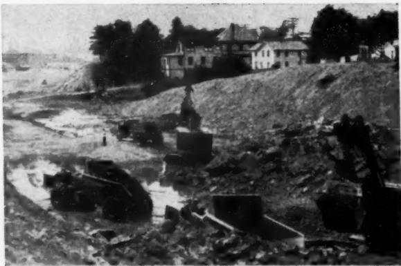
Job No. 1 Cutting 70,000-yd. by-pass for U. S. 1 around New Haven business district, each of these 35 m.p.h. C Tournarockers hauled 600 pay yds. of sandstone per day on 2000' cycles. Entire job was only 1700' long, with all excavation made at this end of the area.
